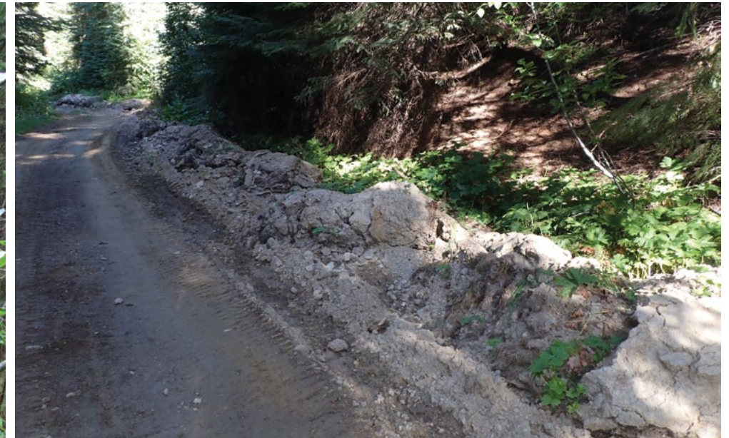
Picture of a berm of dirt (above) moved to the side of FSR 1826, suggesting, with tracks, the presence of heavy machinery on this road prior to any project authorization.
